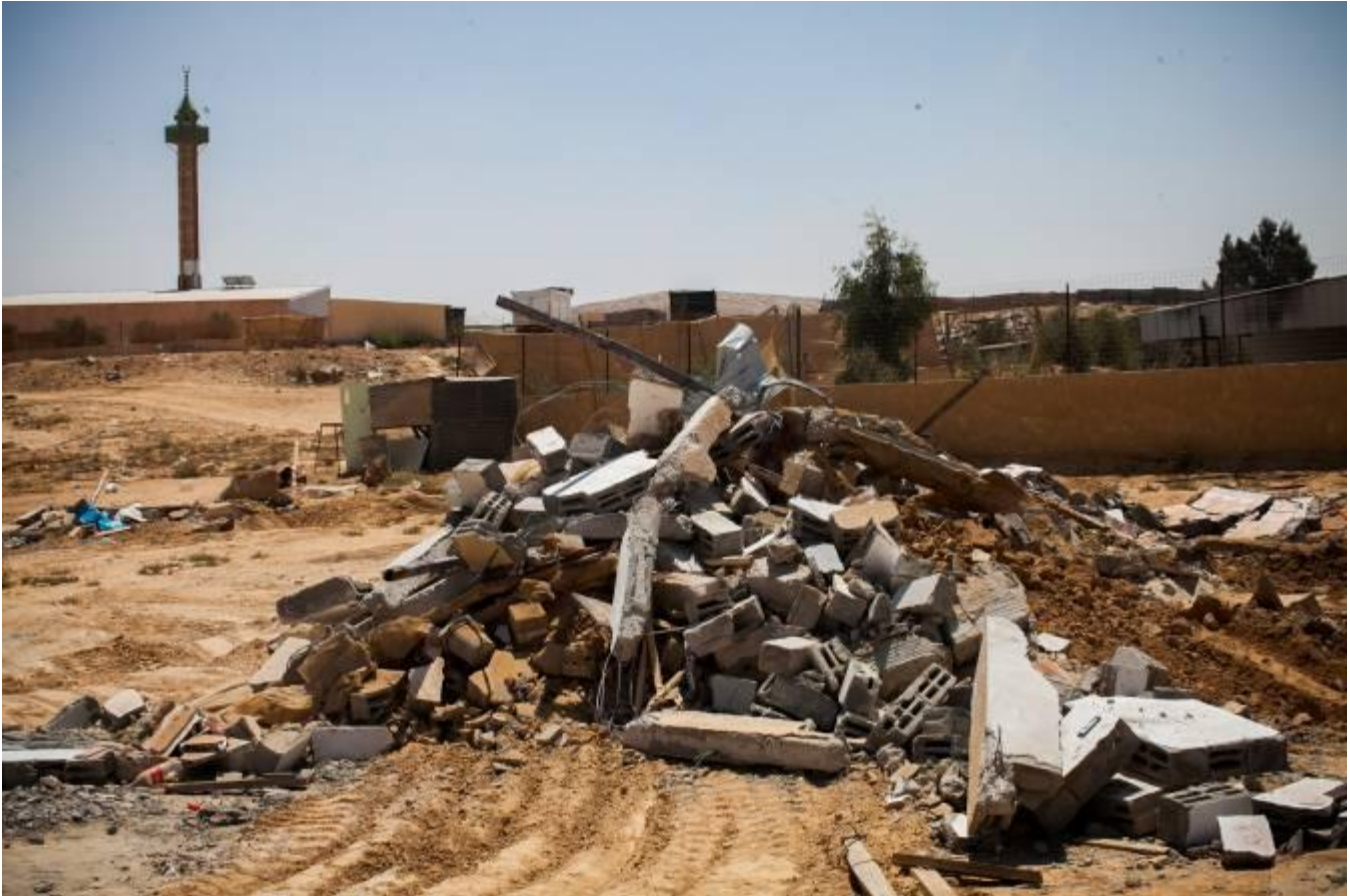
House ruins in the Bedouin recognized village of Kaser a-Sir, August 26, 2013. Photography: Activestills
